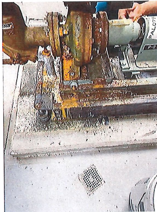
Figure 01: Existing Chilled Water Pump
