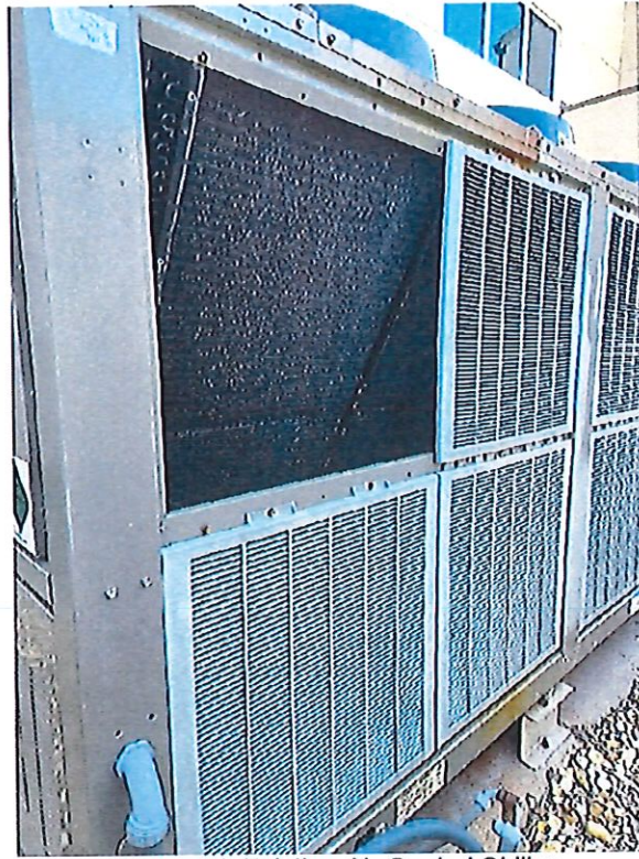
Figure 04: Existing Air-Cooled Chiller
