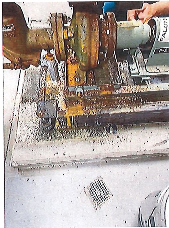
Figure 01: Existing Chilled Water Pump
