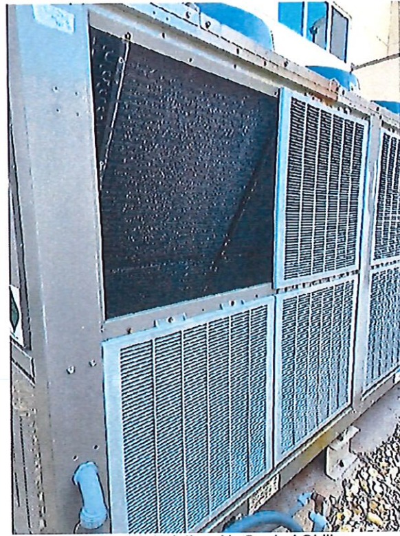
Figure 04: Existing Air-Cooled Chiller
