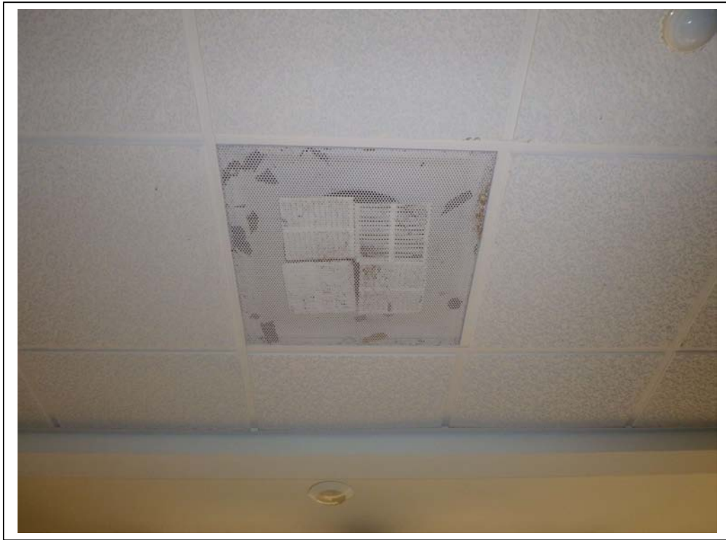
Photo #13; Dusty/Moldy Supply Air Diffuser View
