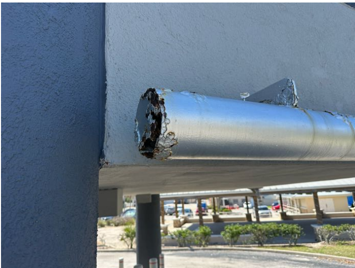
Rust on exterior metal component
