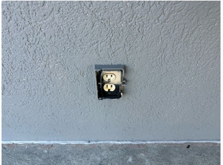
Missing cover on exterior electrical outlet
