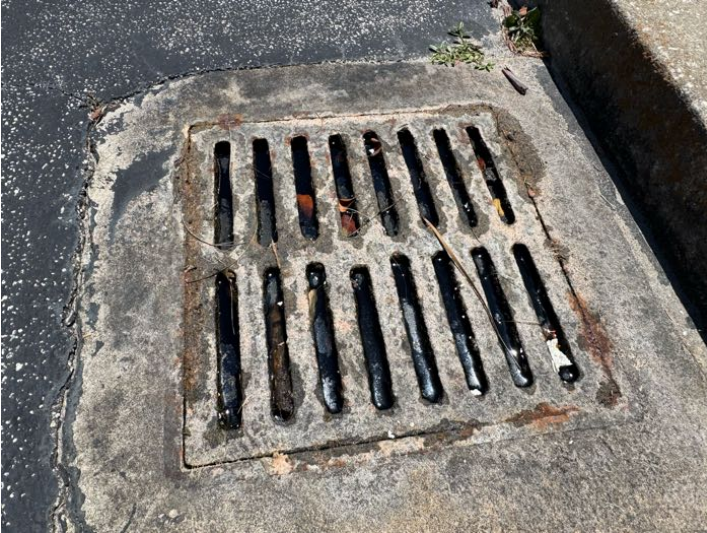
Drainage grate filled with water
