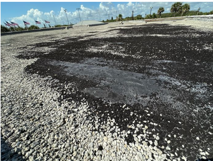
Large area of missing gravel on the roof
