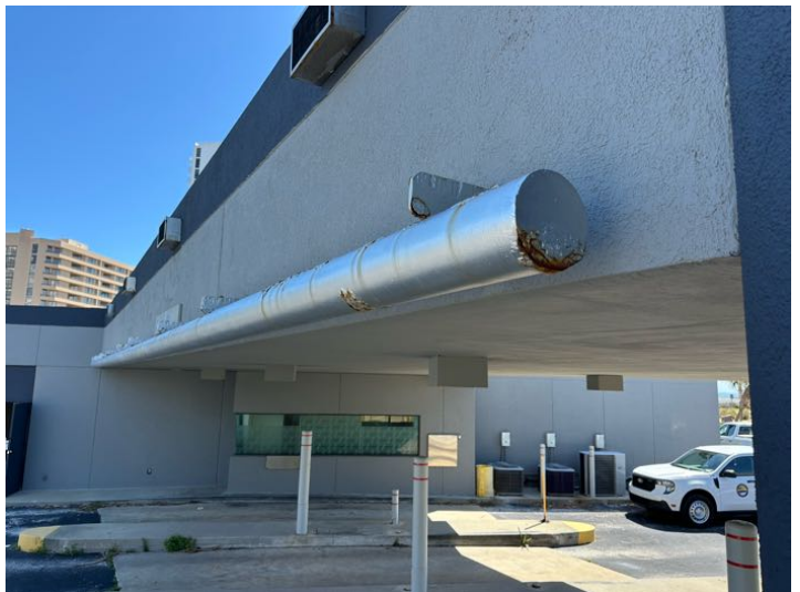
Rust on exterior metal component
