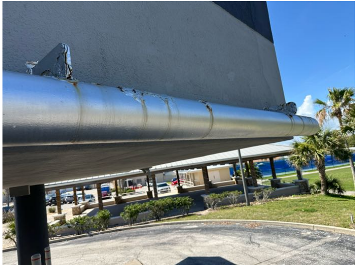
Rust on exterior metal component
