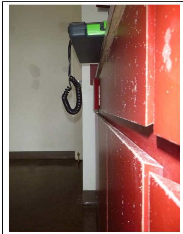
Photo #16; Break Room – Moldy Cabinets View
