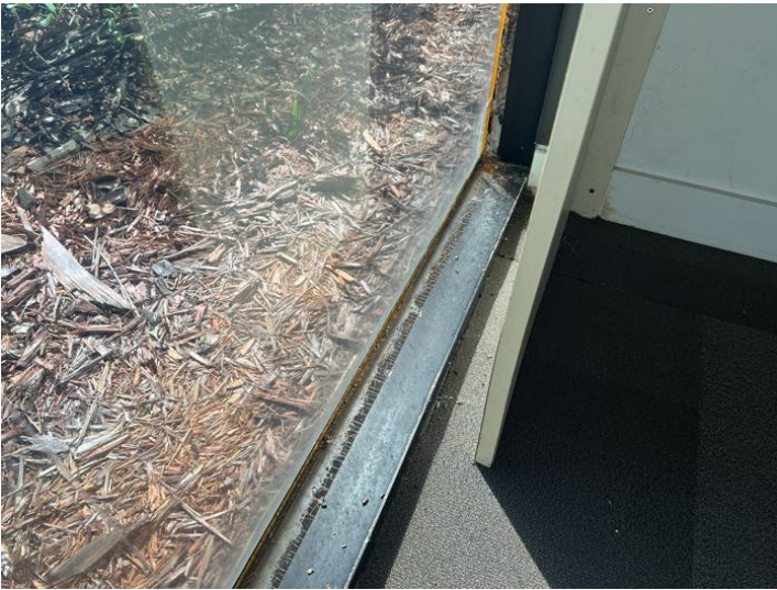
Window seal appears to be failing
