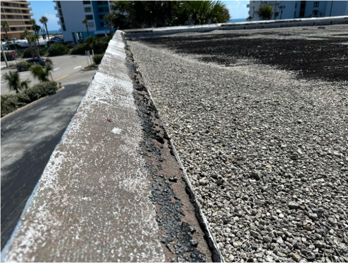
Damage to parapet wall cap
