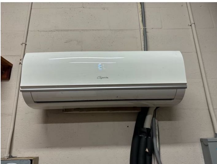
Error code displayed on the mini-split air conditioner unit
