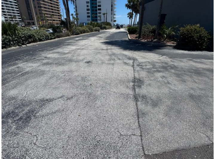
Worn area of parking lot
