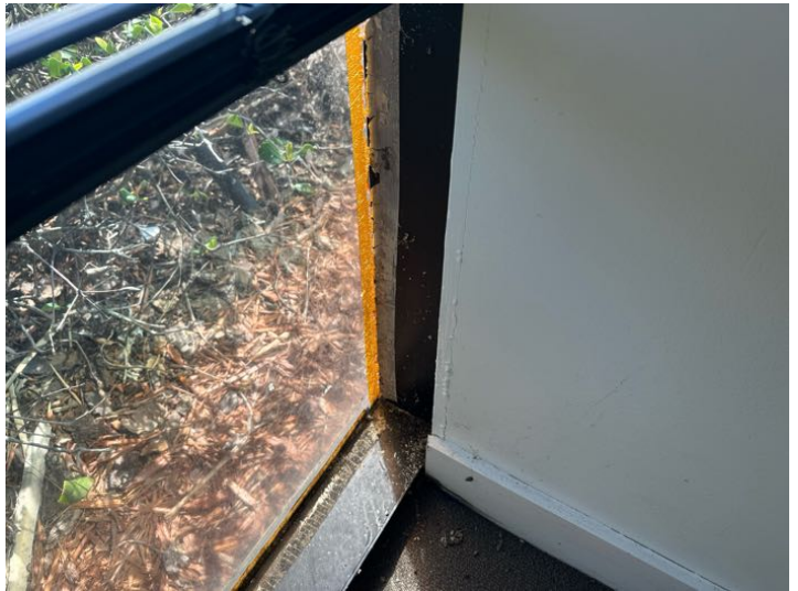
Window seal appears to be failing
