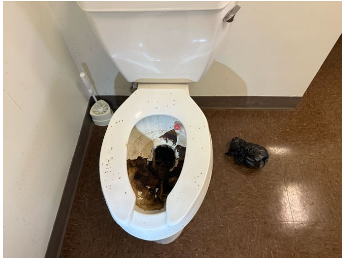
Toilet not tested (no water)
