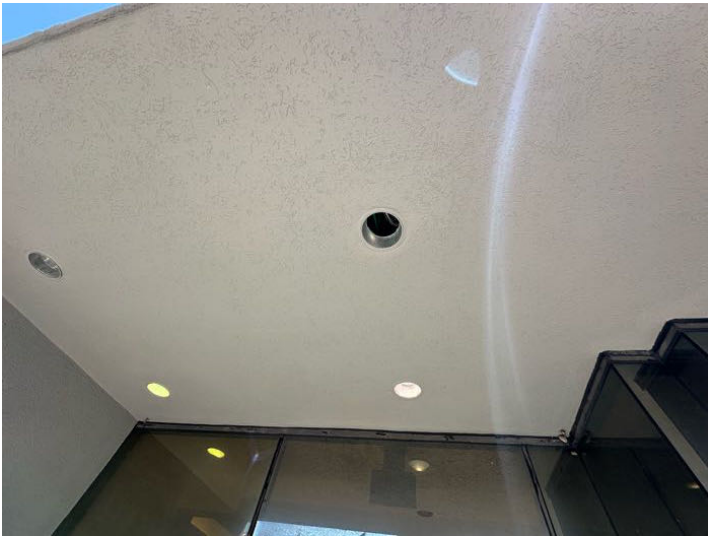
Missing light fixture
