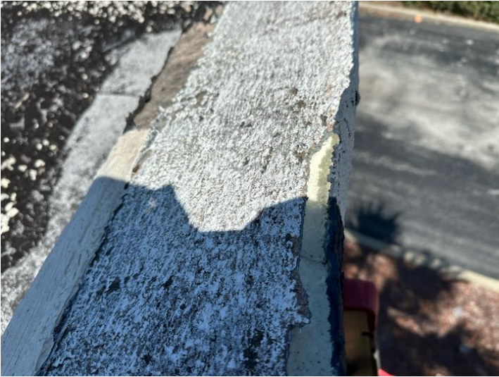
Damage to parapet wall cap
