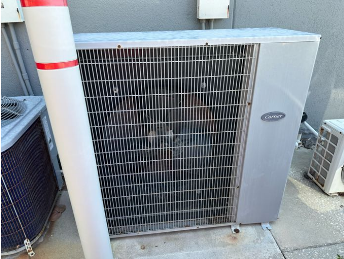
Rusted air-conditioning compressor unit
