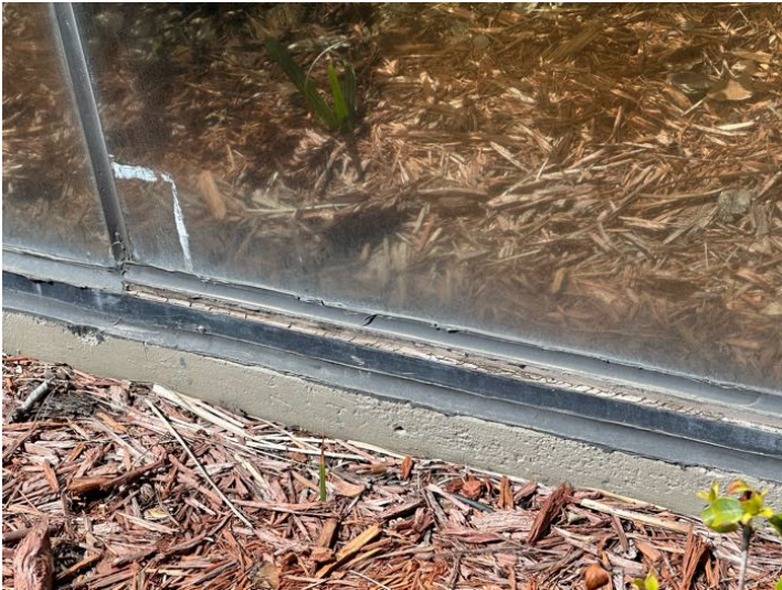
Apparent damage on window seals
