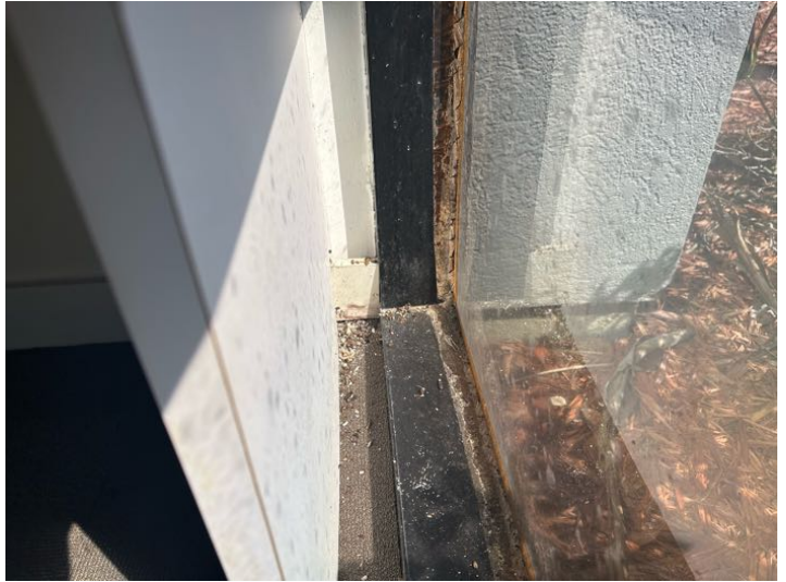
Window seal appears to be failing
