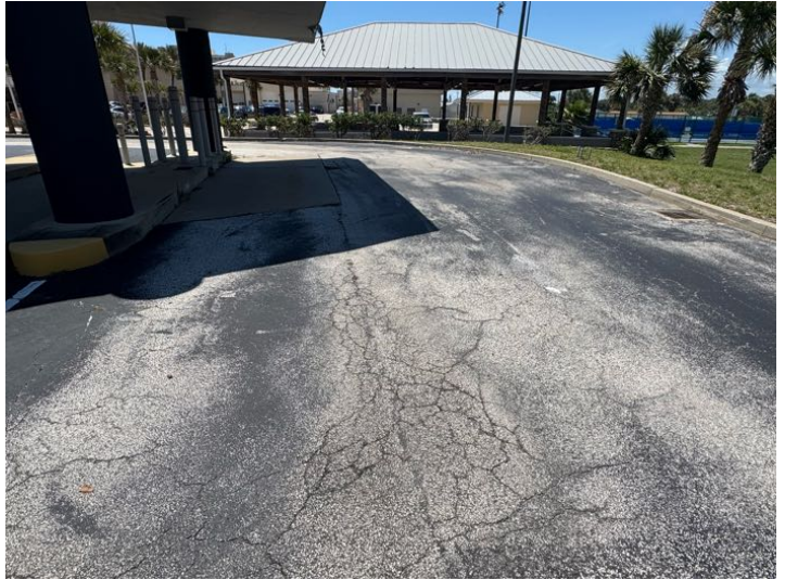
Weathered/worn area of parking lot
