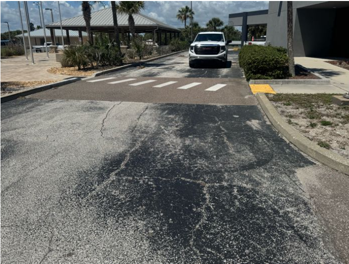
Worn area of the parking lot
