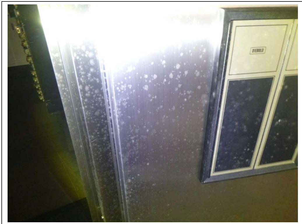
Photo #10; Moldy Vault Door View
