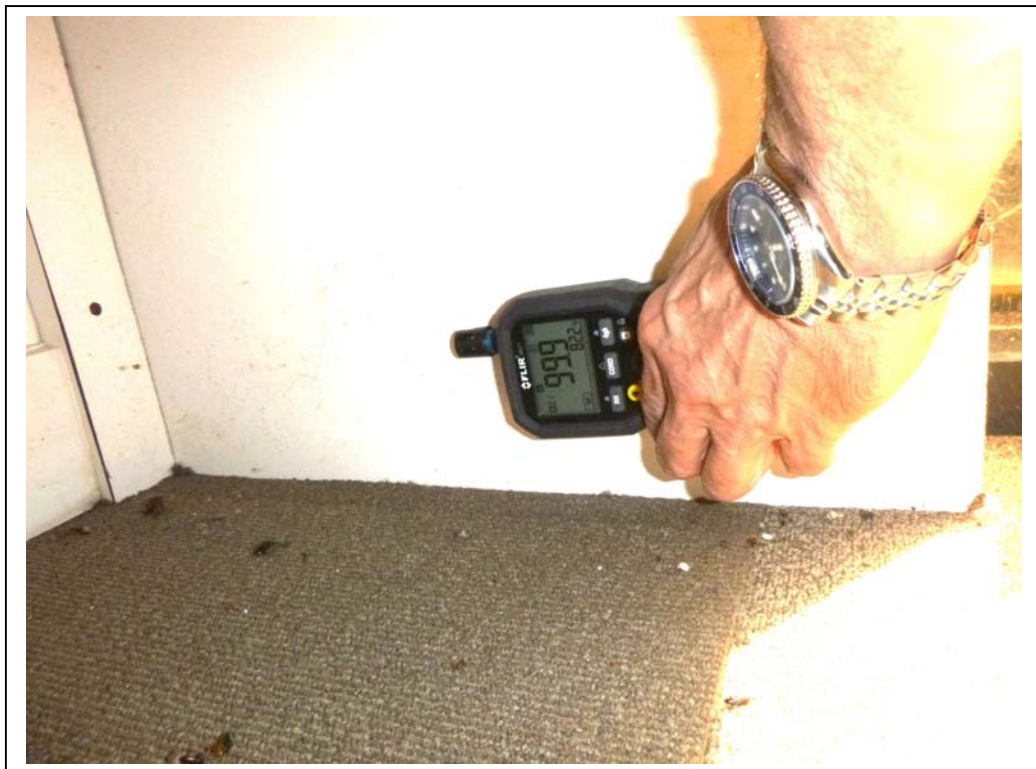
Photo #8; Private Room #1 - Lower Desk Panel (Wet) Surface Moisture Measurement View
