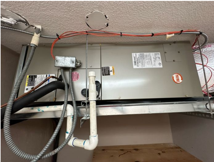
Air handler unit
