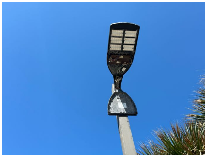
Damaged parking lot light fixture
