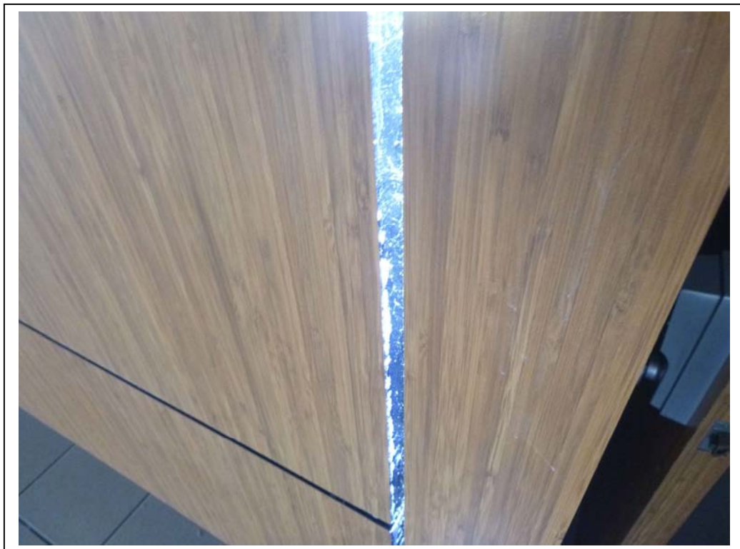
Photo #12; Tellers Desk Side Panel - Moldy Surface View
