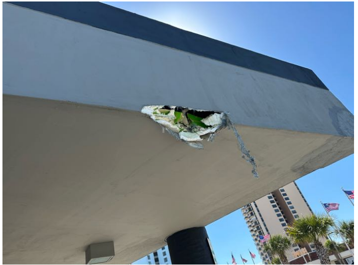
Damage to exterior siding at the drive-through
