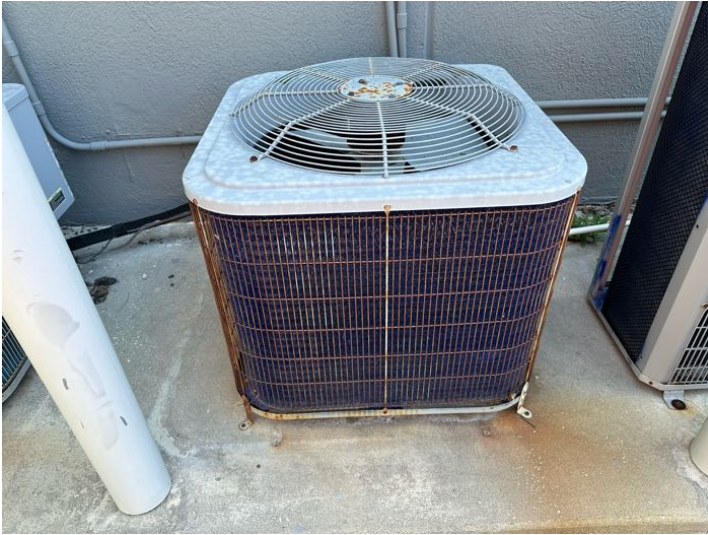
Rusted air-conditioning compressor unit
