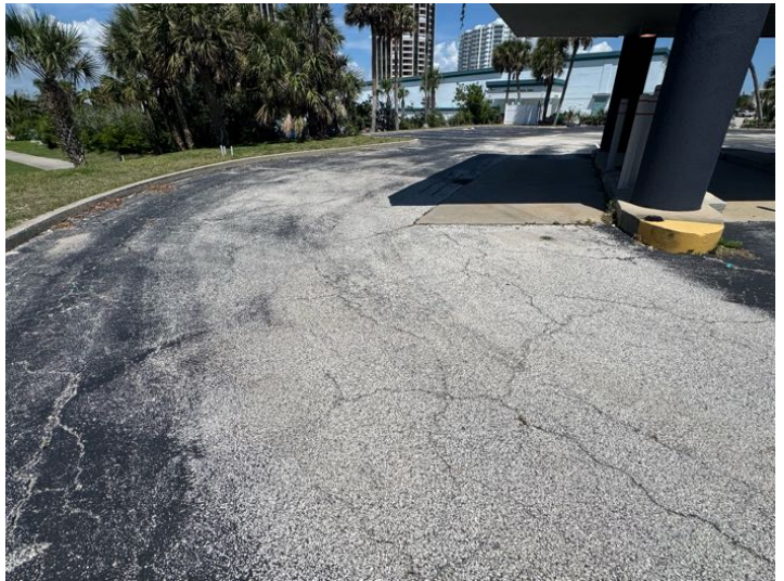
Worn area of parking lot
