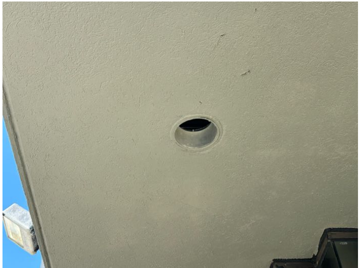
Missing light fixture
