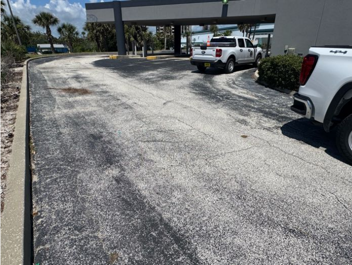
Worn area of the parking lot
