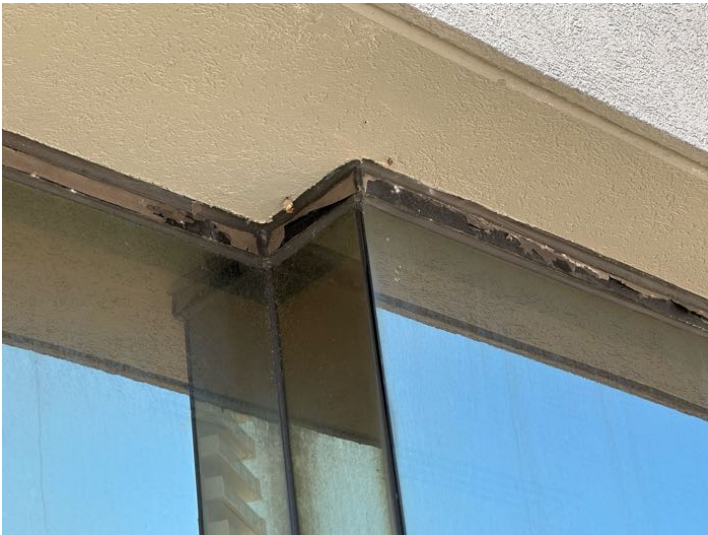
Apparent damage on window seals
