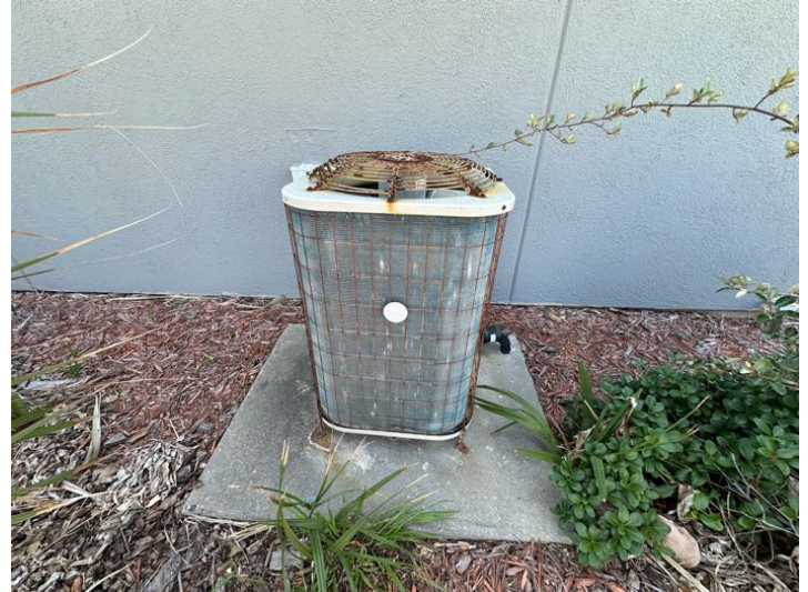
Rusted air conditioning compressor unit
