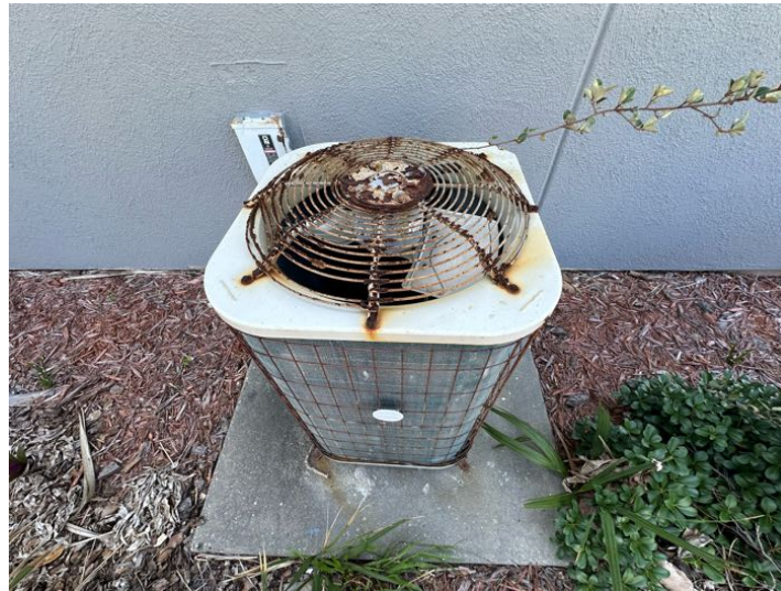
Rusted air conditioning compressor unit
