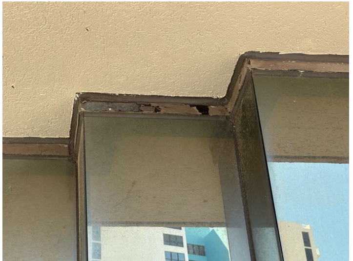
Apparent damage on window seals
