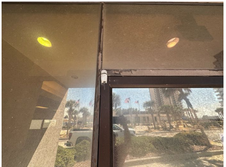
Apparent damage on window seals
