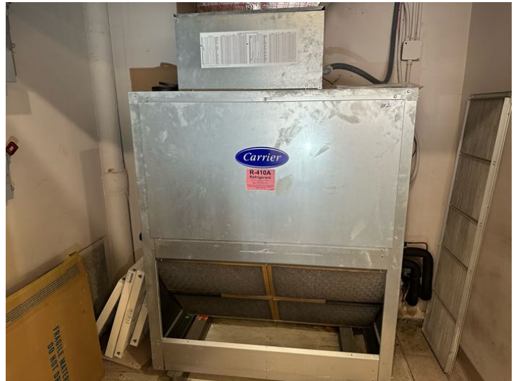
Air handler unit
