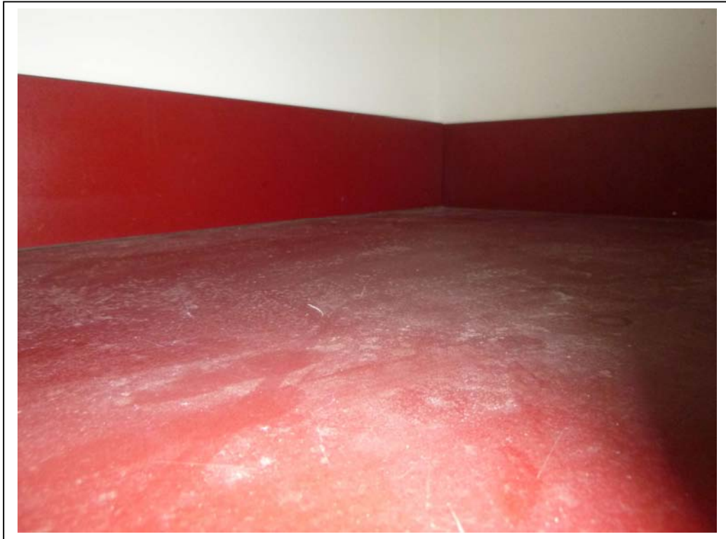
Photo #15; Break Room – Moldy Counter Area View
