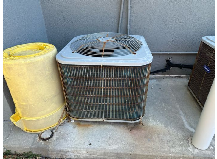
Rusted air-conditioning compressor unit
