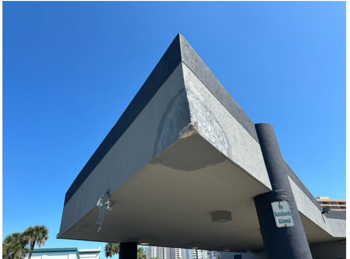
Damage to exterior siding at the drive-through
