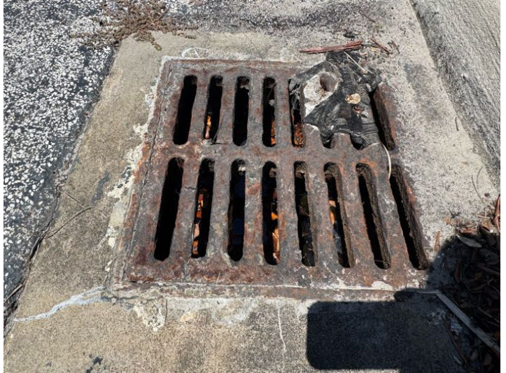
Drainage grate filled with water
