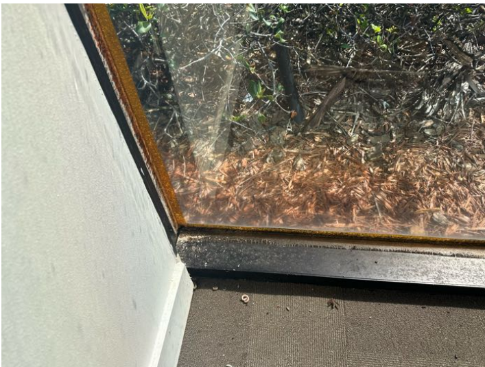
Window seal appears to be failing
