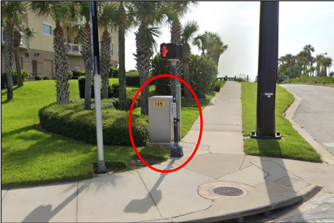
Traffic Signal Control Cabinet: Botefuhr Ave./S. Atlantic Ave.
