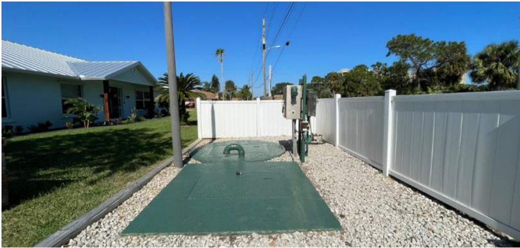
Figure 4-24 Lift Station 10 Photos.
