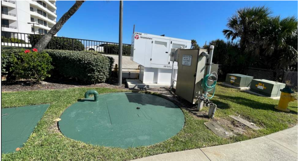
Figure 4-20 Lift Station 8 Photos
