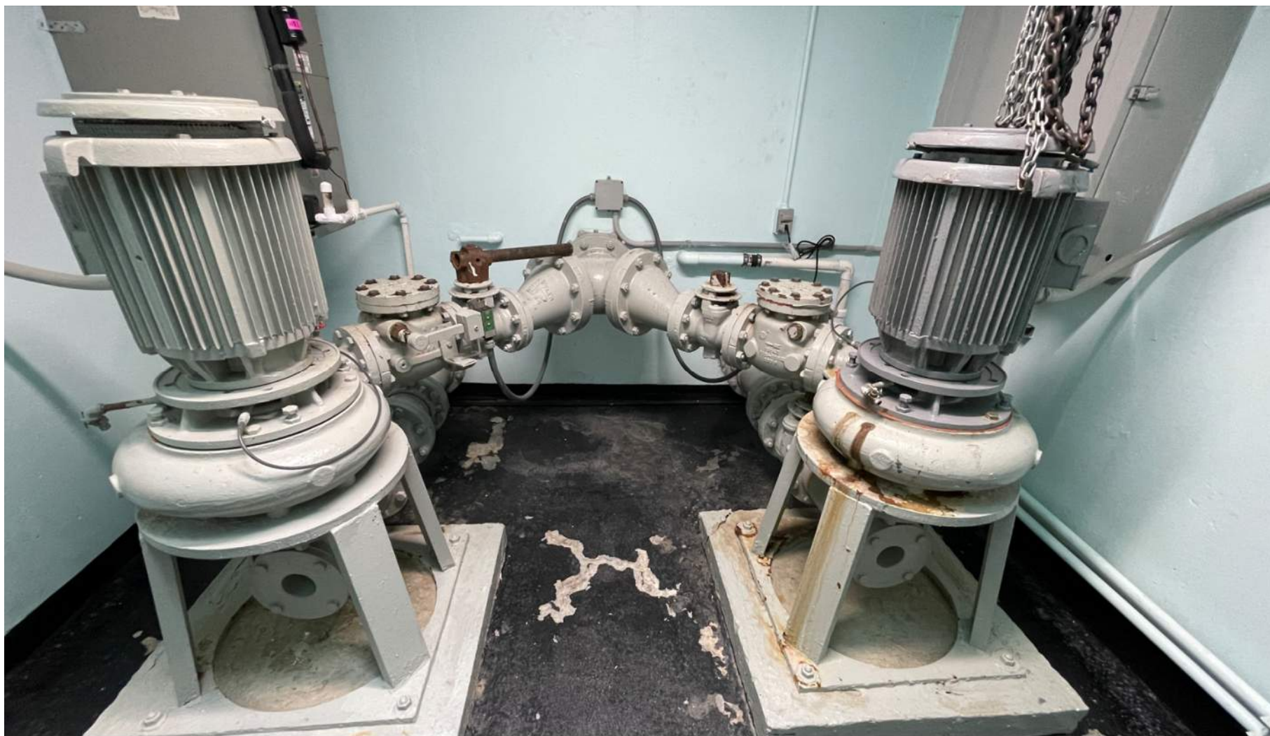
Figure 4-4 Lift Station 1 Dry Well and Pumps
