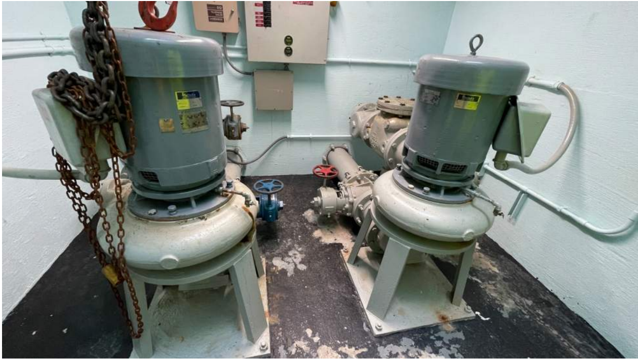
Figure 4-17 Lift Station 6 Pumps
