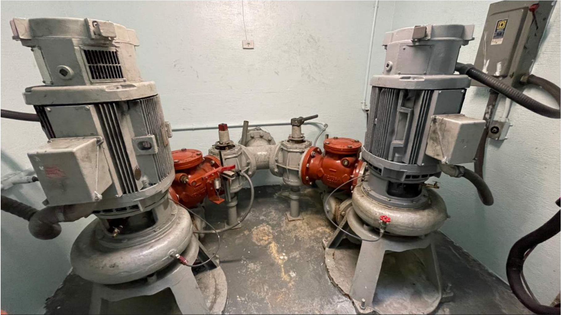
Figure 4-10 Lift Station 3 Dry Well and Pumps
