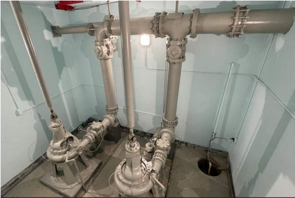
Figure 4-12 Lift Station 4 Pumps and Motors
