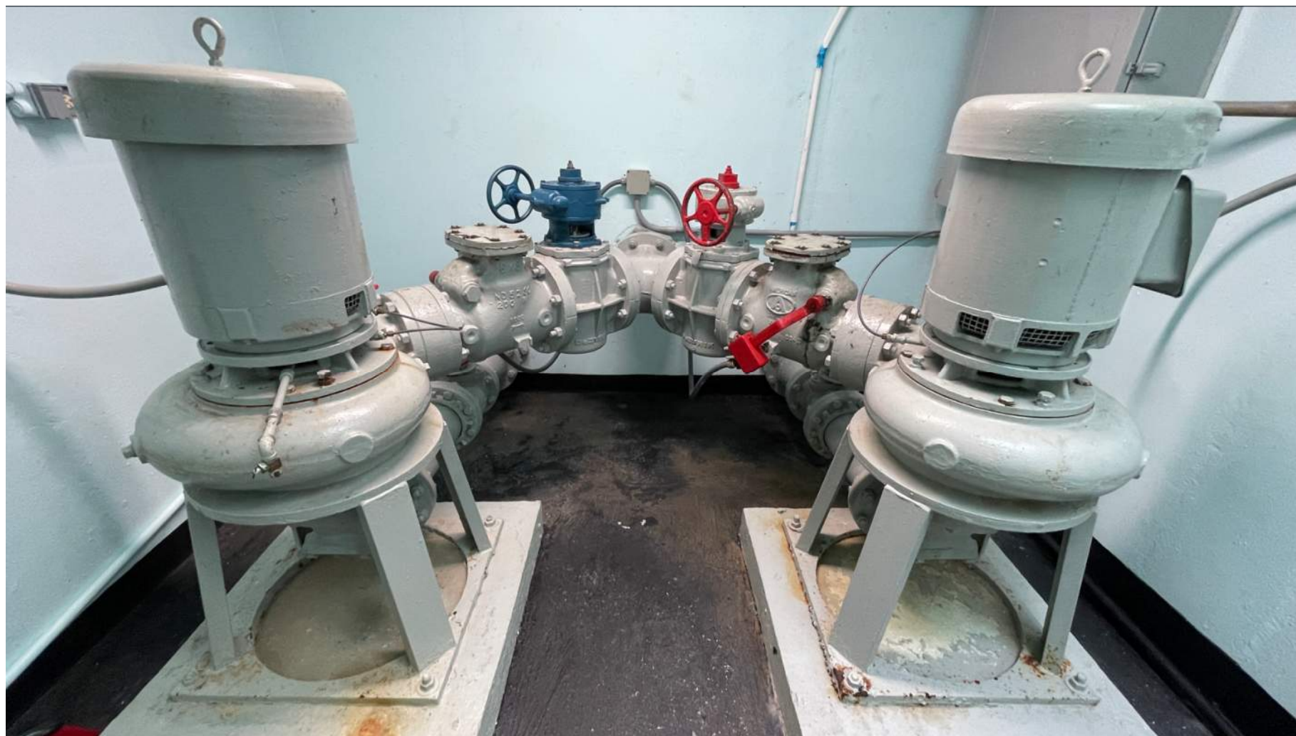
Figure 4-8 Lift Station 2 Dry Well and Pumps
