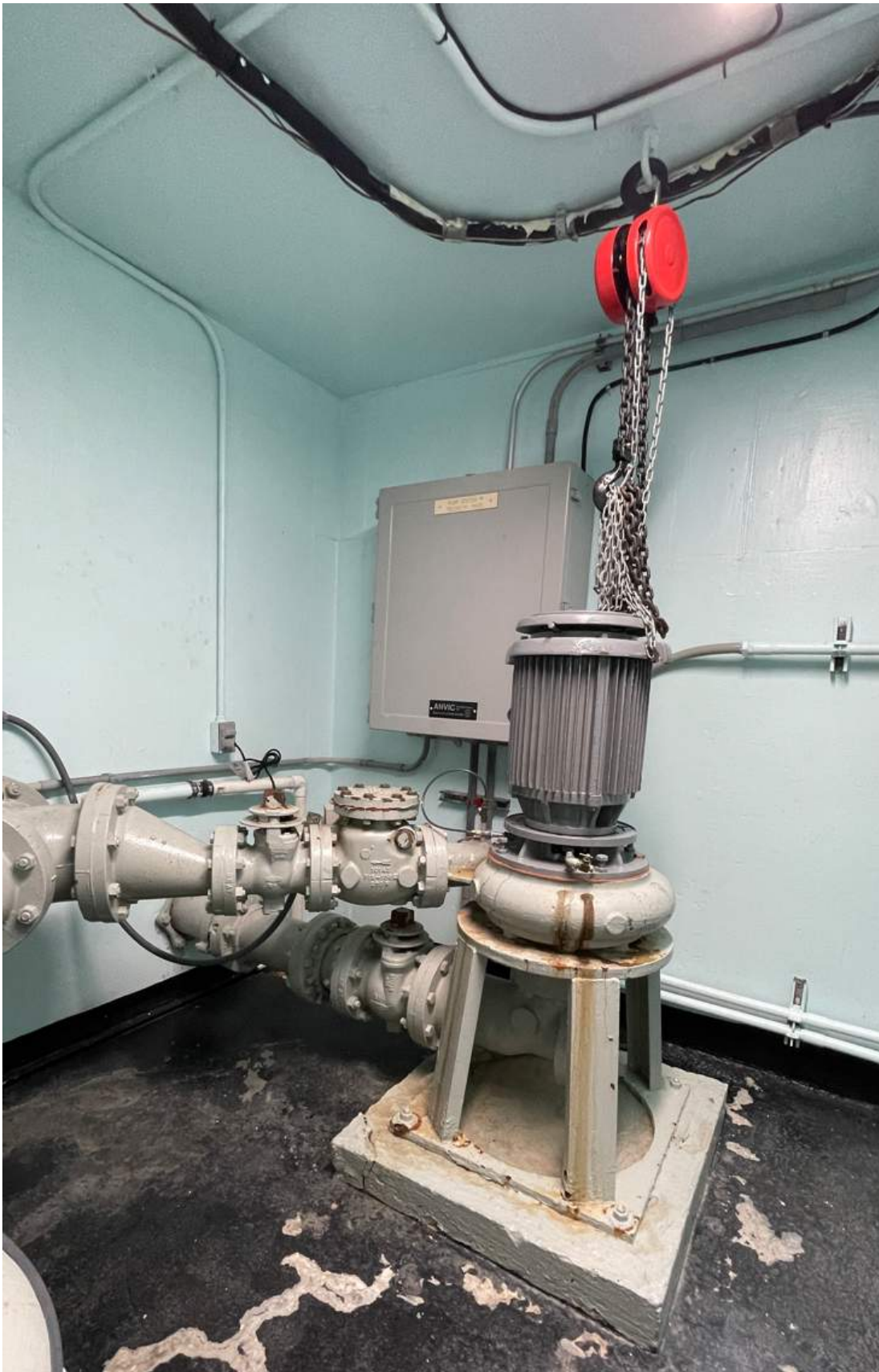
Figure 4-6 Lift Station 1 Pump Lifting Chain
