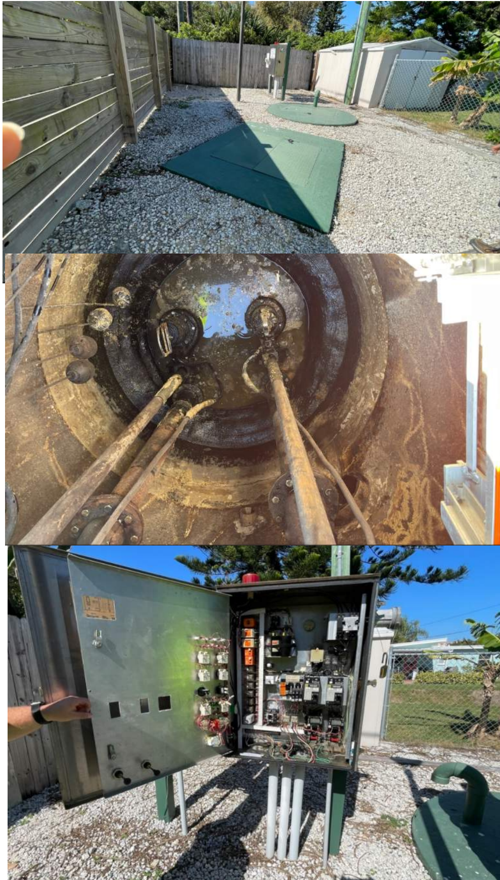
Figure 4-22 Lift Station 9 Photos
