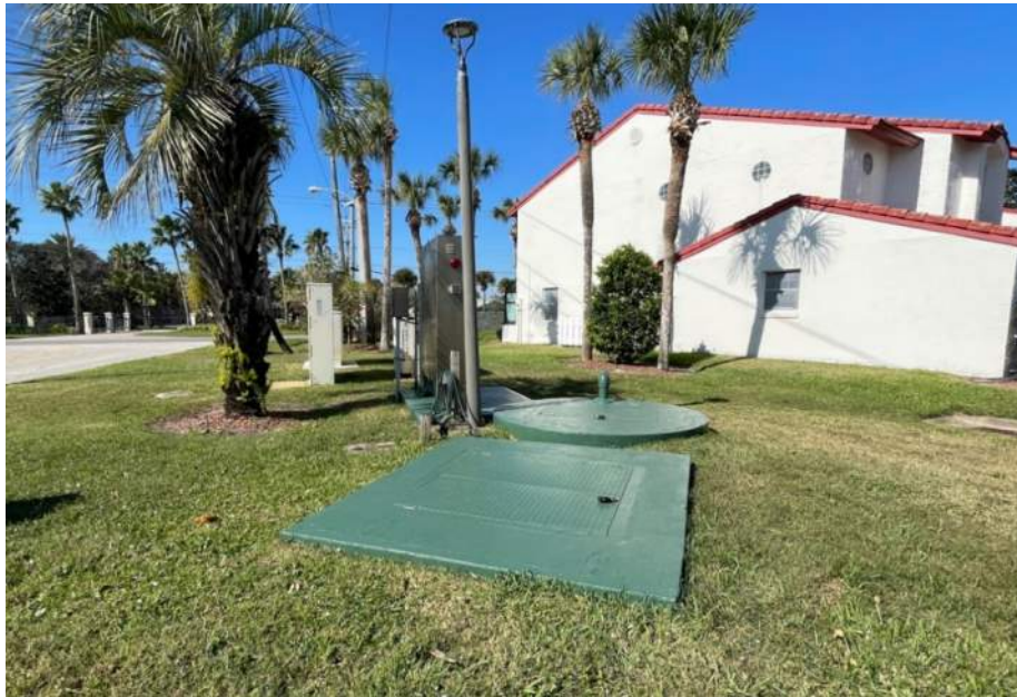
Figure 4-18 Lift Station 7 Photos
